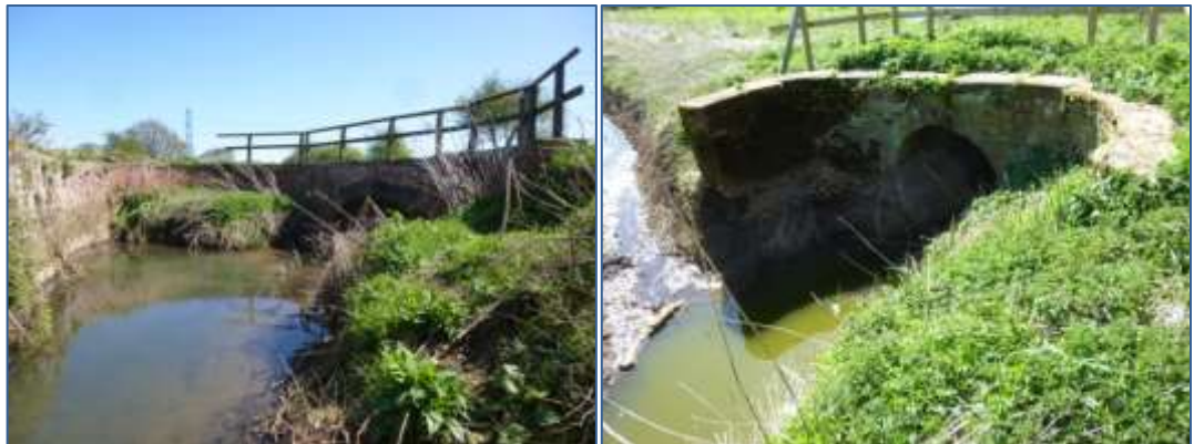
Plates 45-46: Culvert entrances, showing The Beck (HA18; left) and Black Drain (HA27; right)
