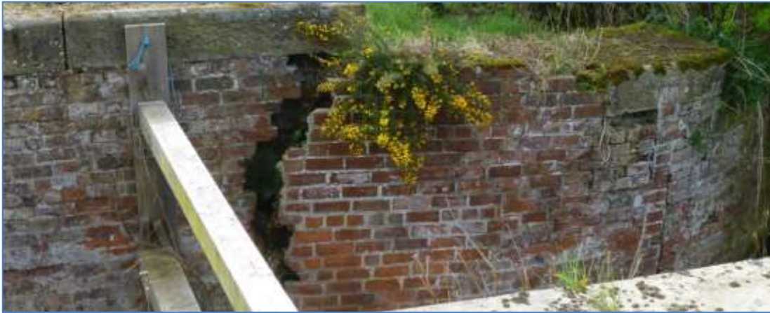
Plate 60: Collapse occurring at Sandhill Lock (HA 8)
