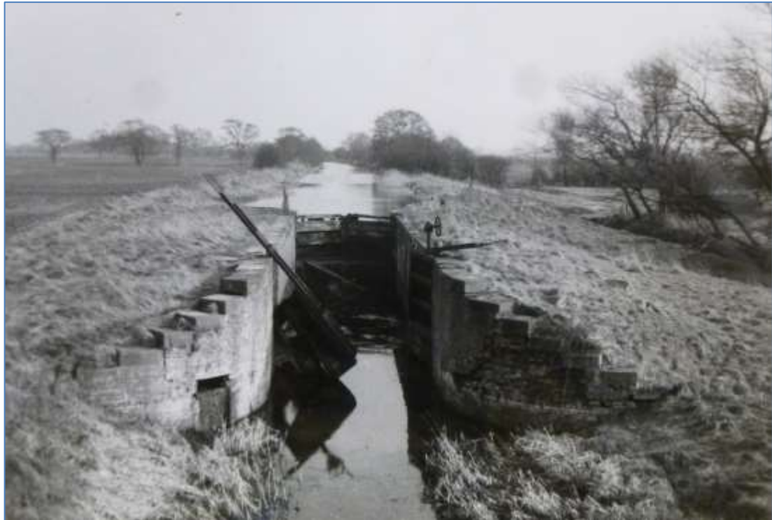
Plate 11: Pocklington Canal in 1959 showing a derelict lock, possibly Walbut (HA 15; © Waterways Museum)
