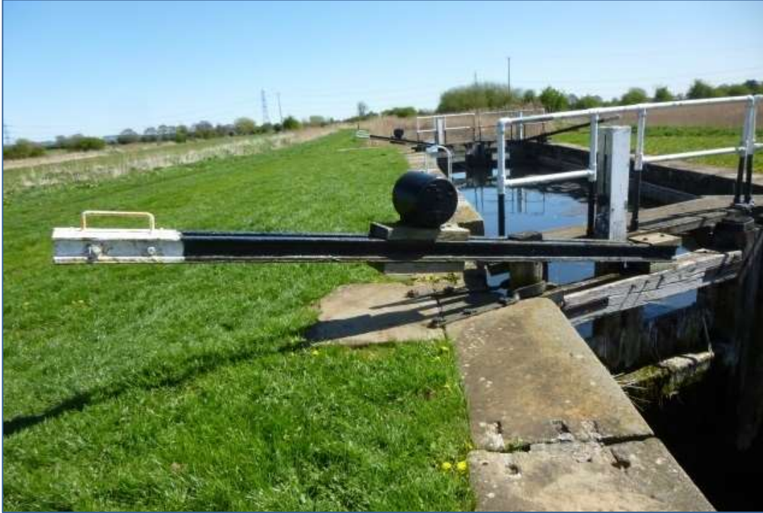
Plate 12: Railway line balance beam with hydraulic paddle gear at Thornton Lock
