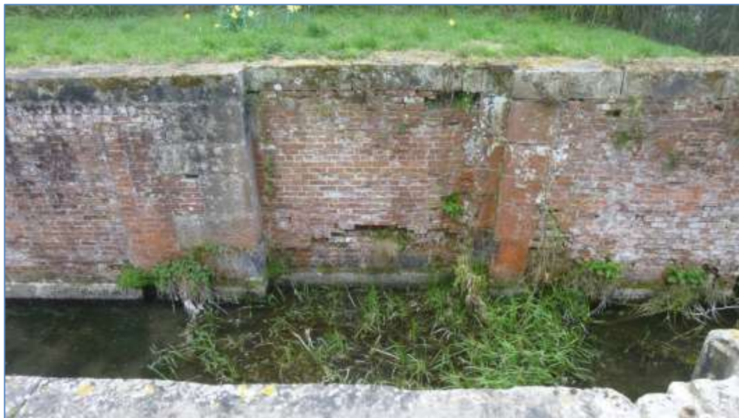
Plate 61: Detail of vegetation damage to Giles Lock (HA 6)
